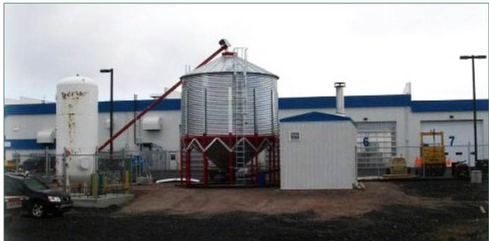
FIGURE 6-4 Biomass fuel storage and boiler at Yellowknife airport (source: Government of the Northwest Territories)
